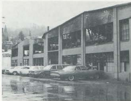
A front view of Wade Mfg. Co.'s central production building, gutted by fire.
